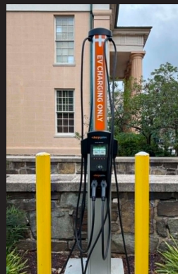
Example of an electric vehicle charging station.
