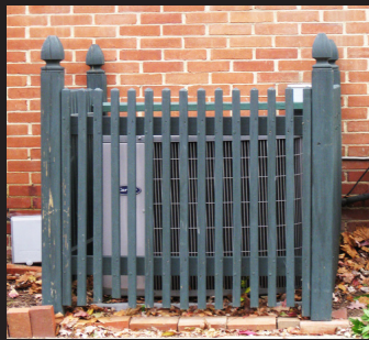
Example of appropriate ground-mounted HVAC screening.
