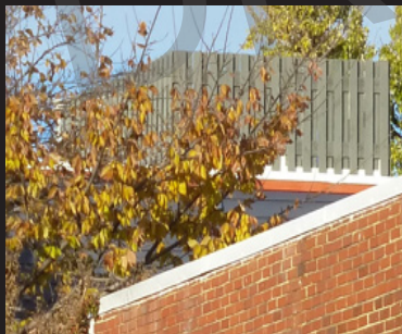
Example of appropriate roof-mounted HVAC screening.
